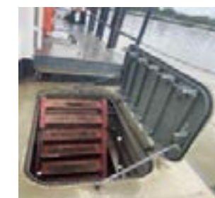
WTC once installed from Top
