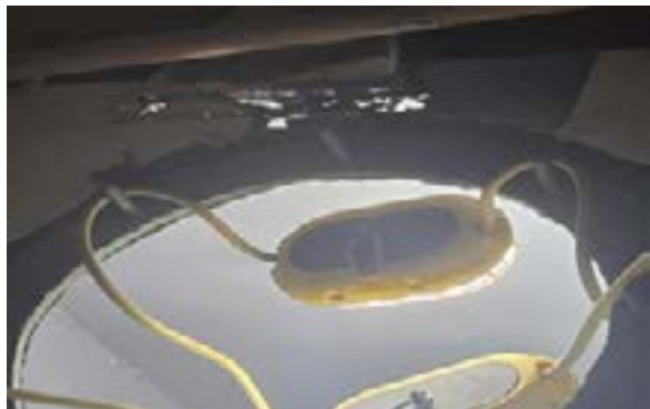
Tank top metal deterioration
