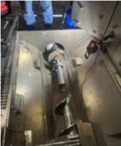
Newly installed Auger shaft/bearing
