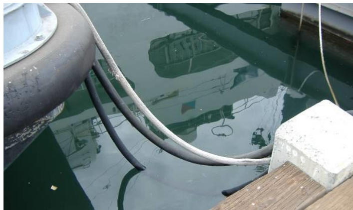
FIGURE 5 – INADEQUATE CABLE SUPPORT AND UNACCEPTABLE SUBMERGENCE
