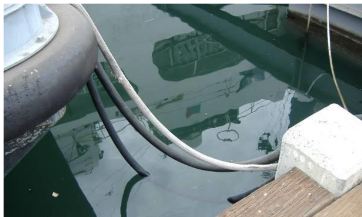
FIGURE 5 – INADEQUATE CABLE SUPPORT AND UNACCEPTABLE SUBMERGENCE
