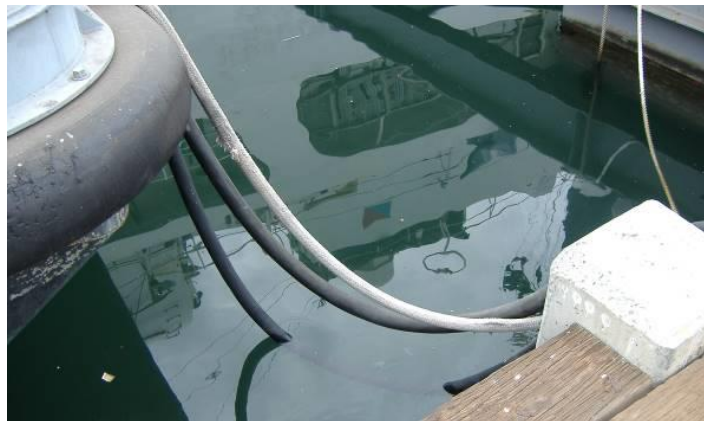
FIGURE 5 – INADEQUATE CABLE SUPPORT AND UNACCEPTABLE SUBMERGENCE
